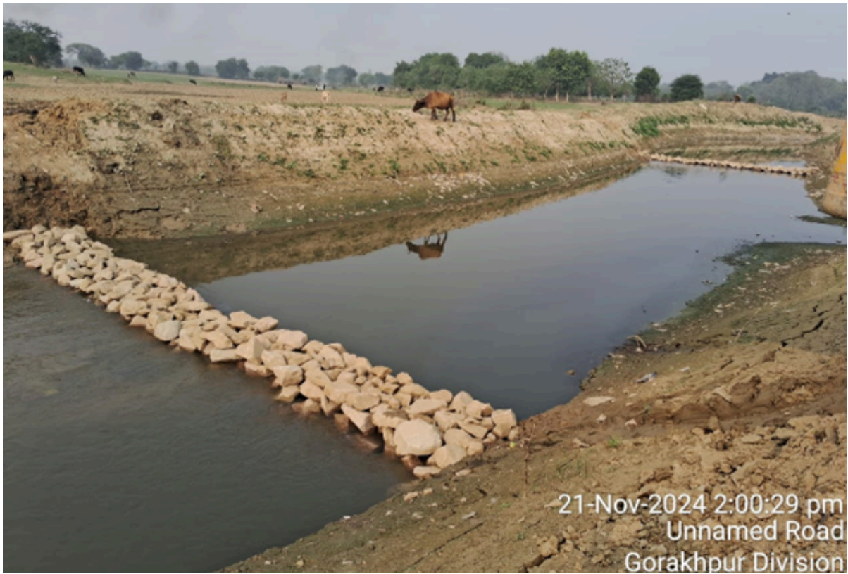
Tertiary drain (Tokia drain) showing the rock filters
